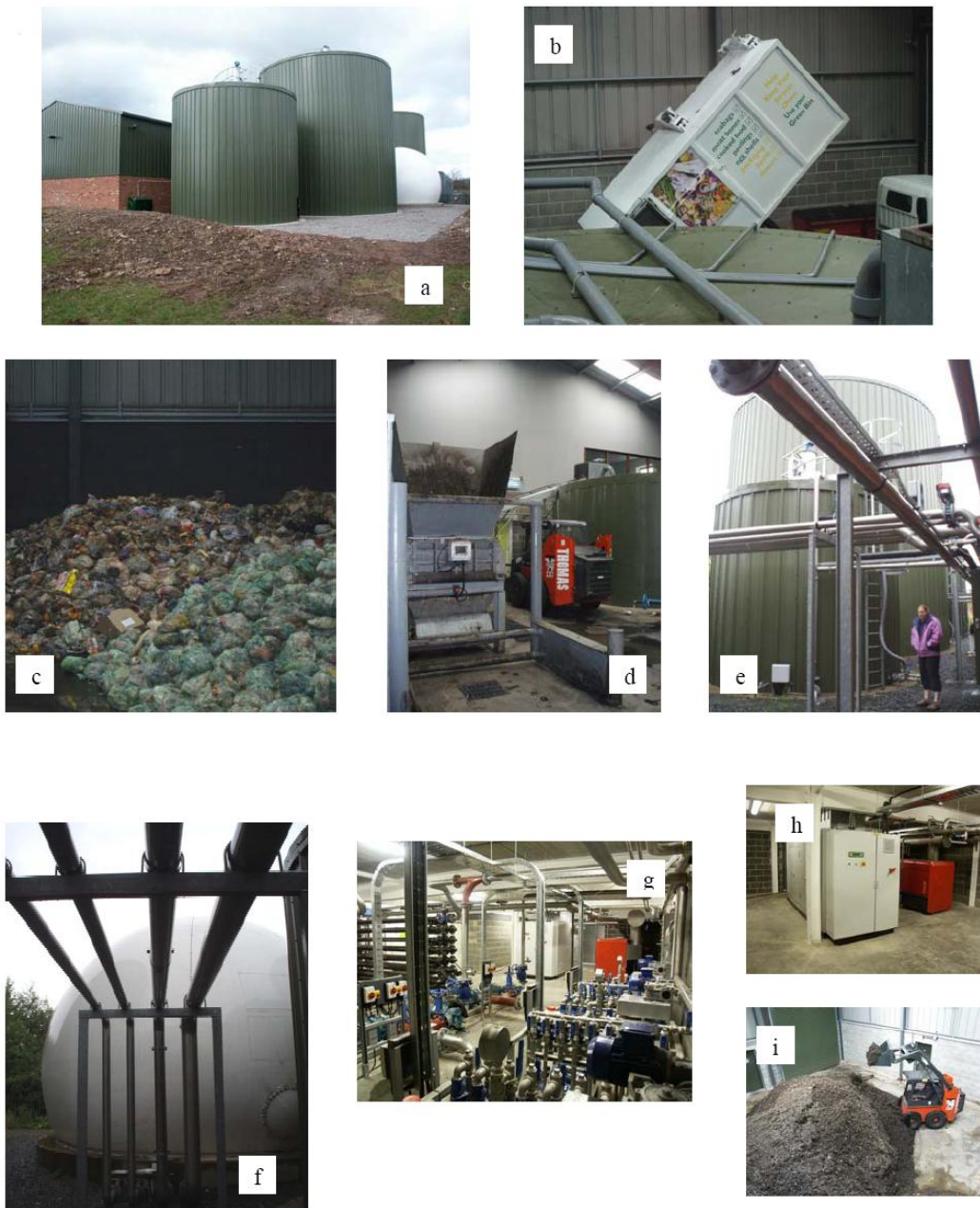
Fig 5.2 The South Shropshire Biogas digester a) building and tanks b) delivery lorry c) waste food in biodegradable bags d) first hopper / shredder e) 900m 3 digester and smaller pasteurisation tank f) gas holder g) plant room h) CHP engine i) dried digestate
